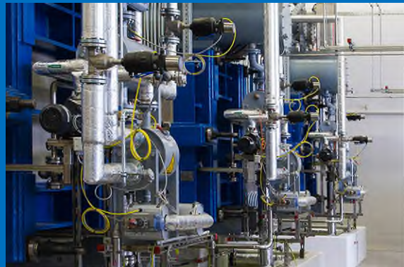
Electrolysis control set-up (Source: Cariboo)
